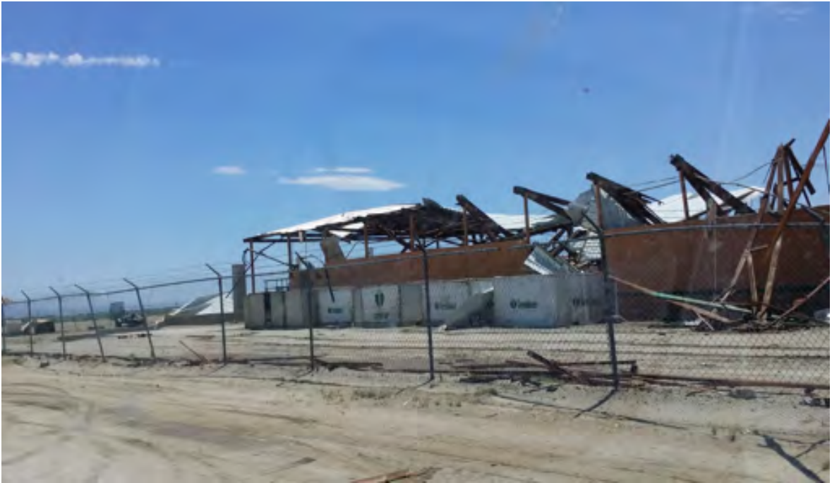
Figure 59. A Roof was Torn Off by the 2015 Tornado.
