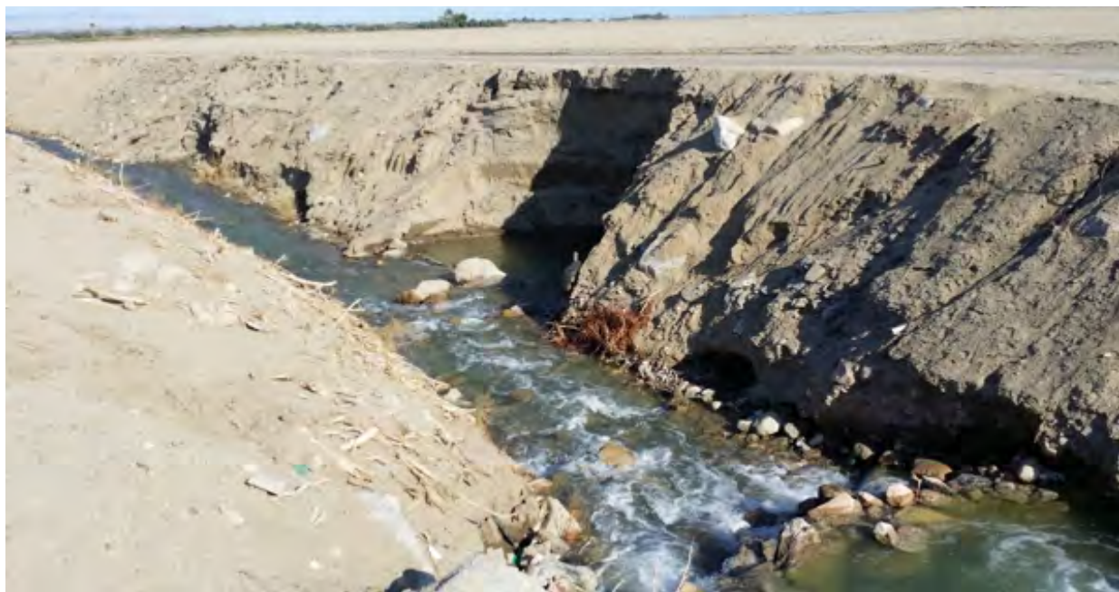
Figure 18. Avenue 68 Undermined by the Canal.
