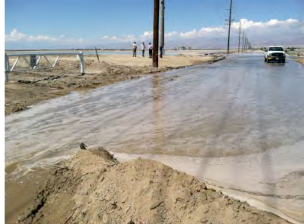
Figure 17. Flooding on Fillmore Street.
