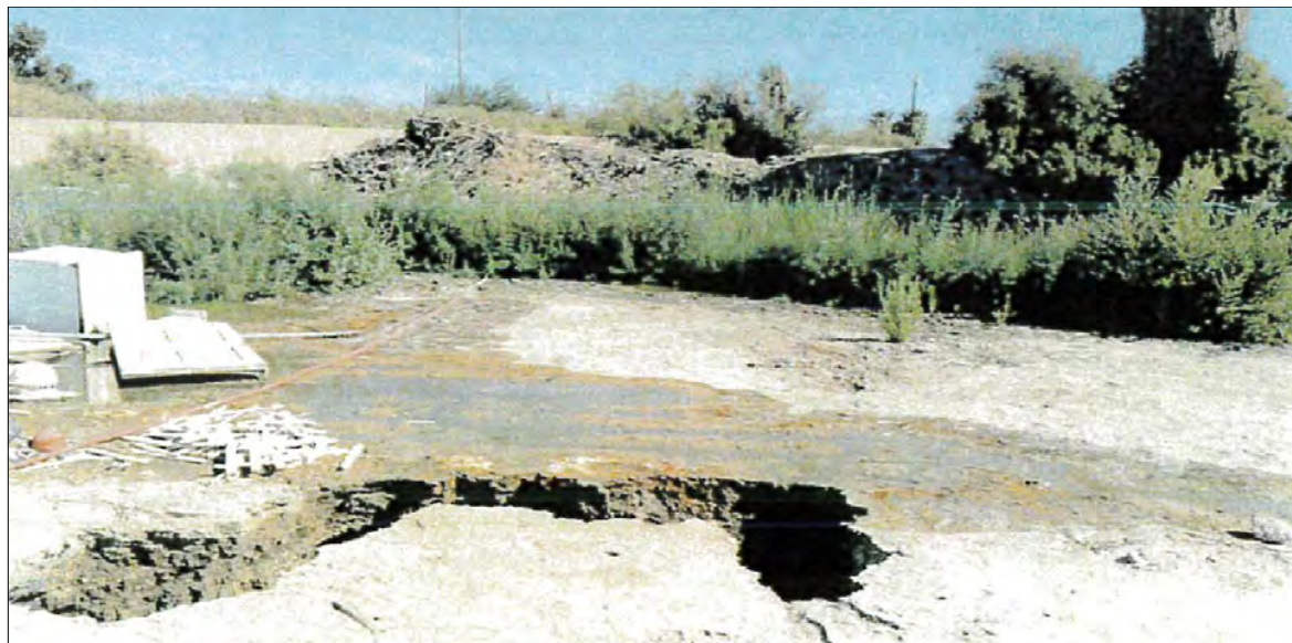
Figure 45. Ground Sinking at an Artesian Well on the Torres Martinez Reservation (Jackson Street, Thermal).
