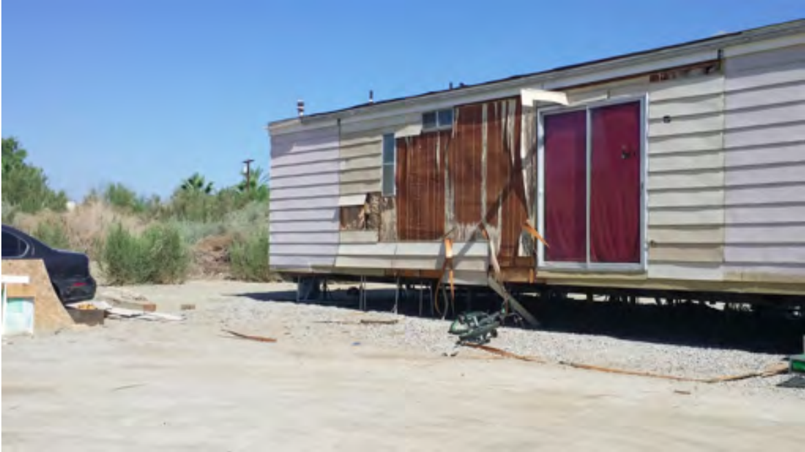
Figure 60. A Mobile Home Sustained Damage from the 2015 Tornado.
