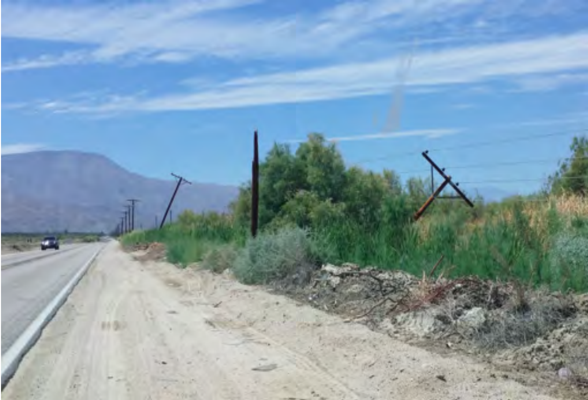
Figure 58. Downed Power Poles from the 2015 Tornado.
